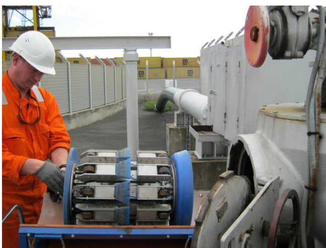
Figure 3. Loading the MFL tool into the trap valve in readiness for launch.
