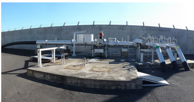
Figure 2. The pipeline departs to the left. The trap valve is in the centre.
