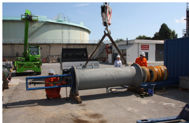
Figure 5. Temporary trap – a pipe joint.
